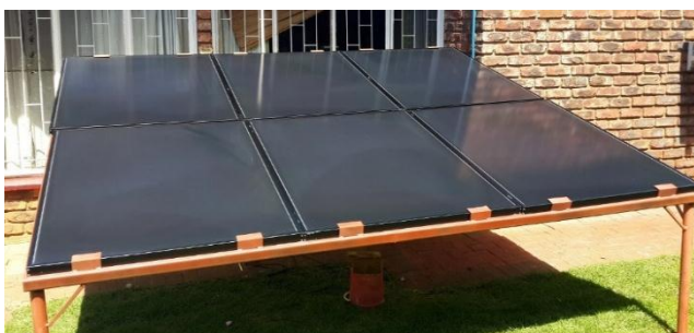
Figure 6. Installed PV modules
