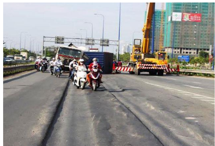
Fig. 1. Longitudinal ruts on asphalt concrete road pavement in Vietnam
