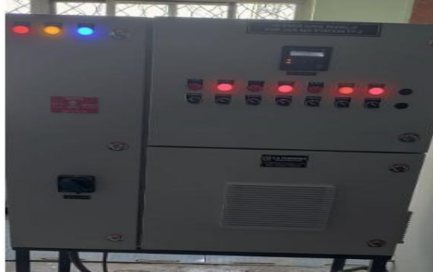
Figure 6: APFC Control and Relay Panel
