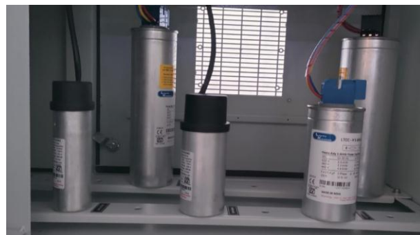
Figure 7: Capacitor Banks of APFC
