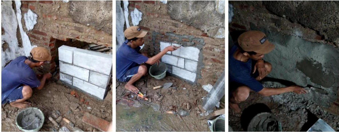
Fig 9. Retrofitting of masonry wall in site – (a) Filling the removed part by concrete bricks; (b) filling the space between new concrete bricks and the old masonry wall; (c) Plastering the retrofitted masonry wall
