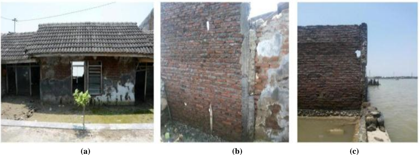
Fig 3. Situation of the site: (a) a house that directly adjacent to the sea; (b) the broken part of clay brick masonry wall; (c) the area outside the house that submerged by seawater and routine tidal flooding
