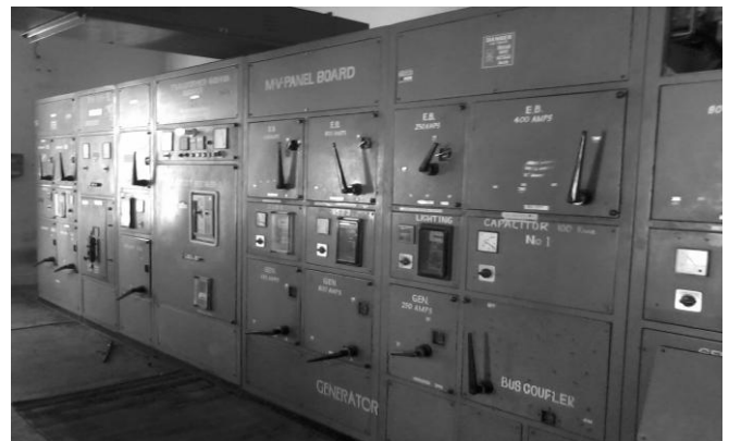
Figure 1 Panel arrangement in the power House
